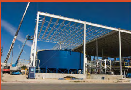
TECHNOLOGY TITANS Samsung Austin Semiconductor makes progress on its $3.6 billion manufacturing plant addition.
